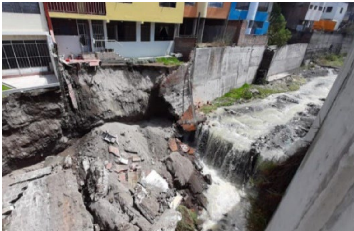
Figure 22. Heavy rains trigger erosion and undermining of the San Lázaro gorge.
