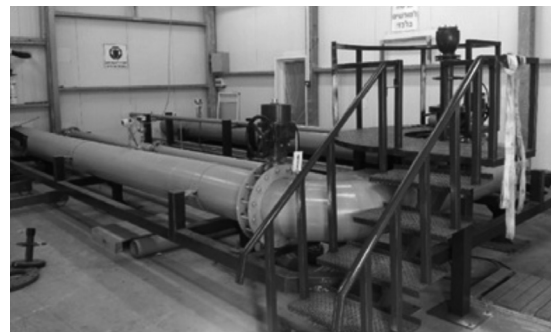
Figure 1. Test bank with Bermad valves.
